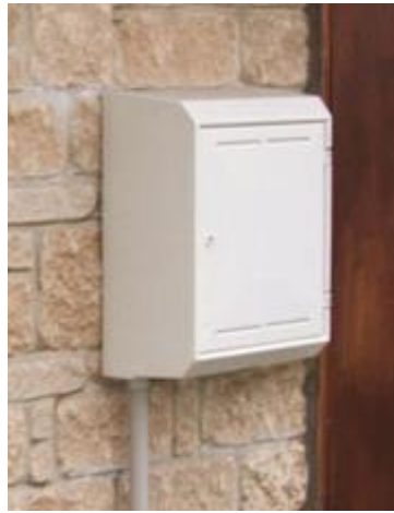
Surface mounted meter box
